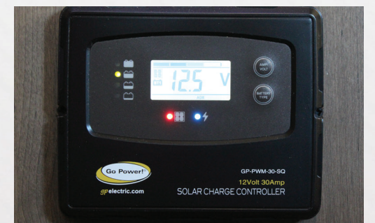
190W Solar Batteries last longer when they are properly charged. A roof-mounted flex panel provides a constant trickle of free power.
